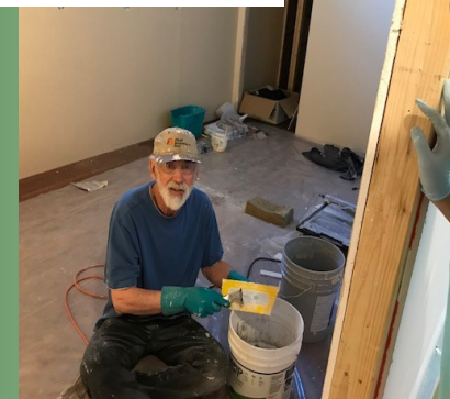
One of our lead volunteer renovators, Ron Olsen, is seen cleaning his trowel after laying dressing rooms and bathrooms flooring
